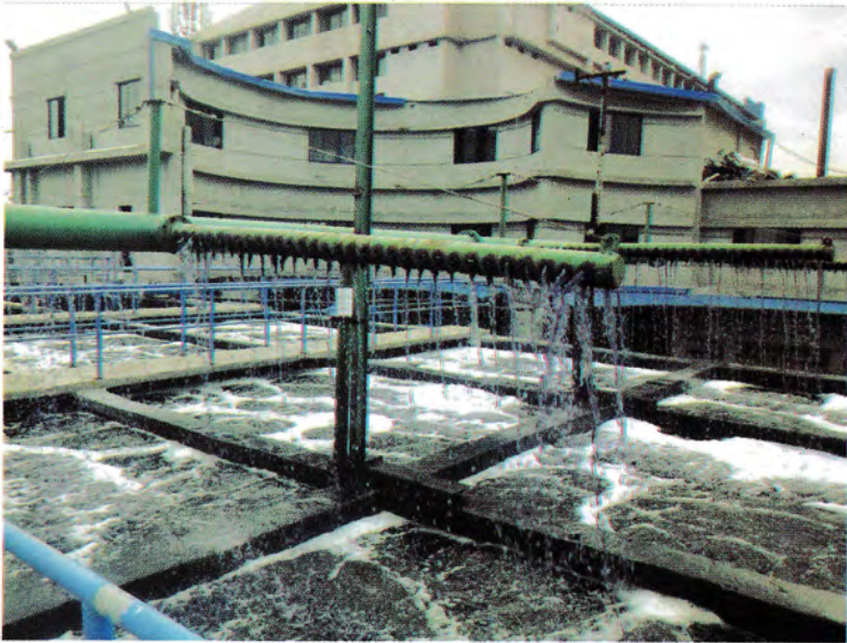
Modern ETP was set up at Aboni Textiles Limited in 2009 is treating wastewater
